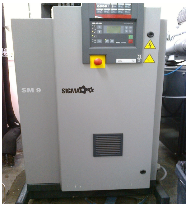
Figure 3. The air compressor
