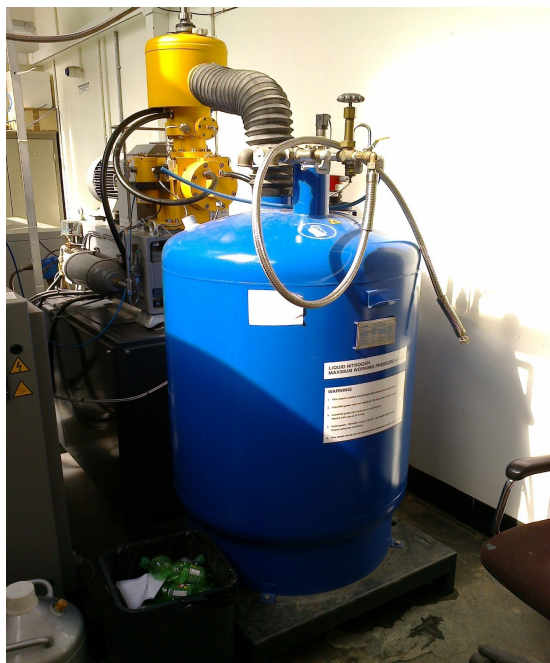
Figure 6. The storage tank
