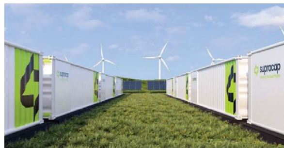
An integrated solar, wind and supercapacitor energy storage 2 MW site in Turkey.
